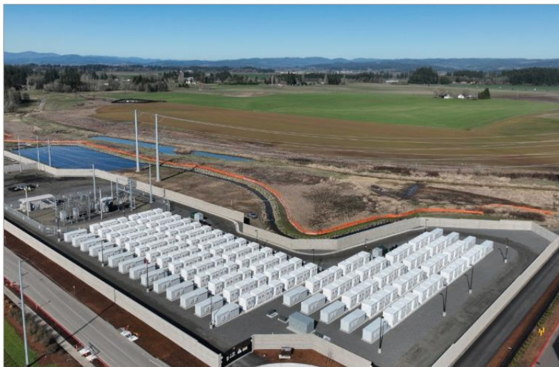
Constable, a PGE-owned facility located in Hillsboro, Oregon. Source: PGE
