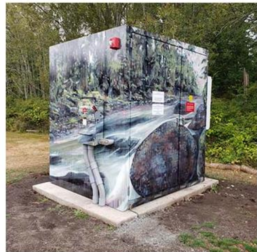
Samish Island Fire Station BESS. Source: PSE
